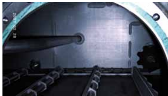
Screening tank, interior view
