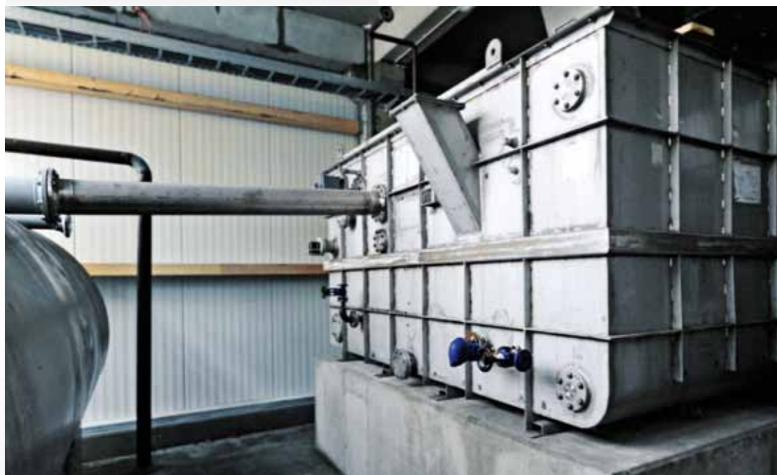
Screening tank, exterior view
